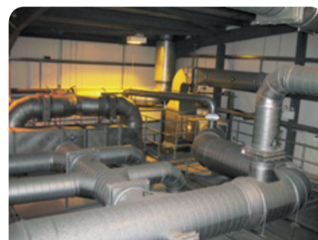
NSG will be on site at LLWR in early 2012 and will begin to remove the contaminated ductwork from within the facility.
